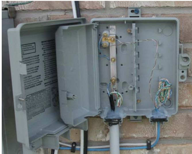
Figure 4. Typical NID (FTTN mode) (our installation)
