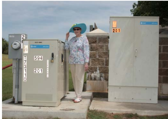
Figure 3. VRAD (l.) and SAI cabinet (r.) (serving our installation)
