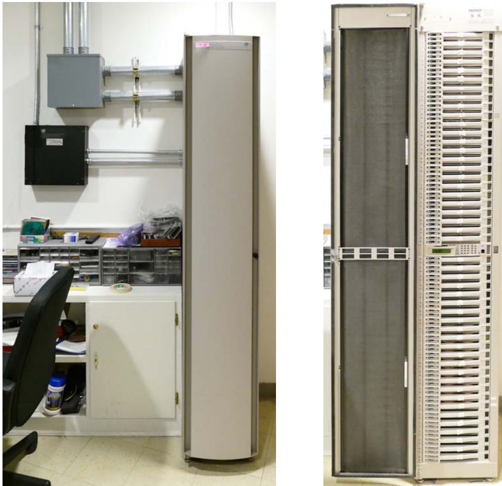
Figure 1. The TEC Sensor SR48 dimmer rack
