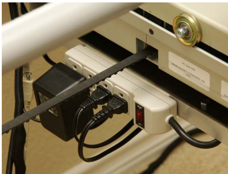
Figure 10. Carriage AC power distribution strip
