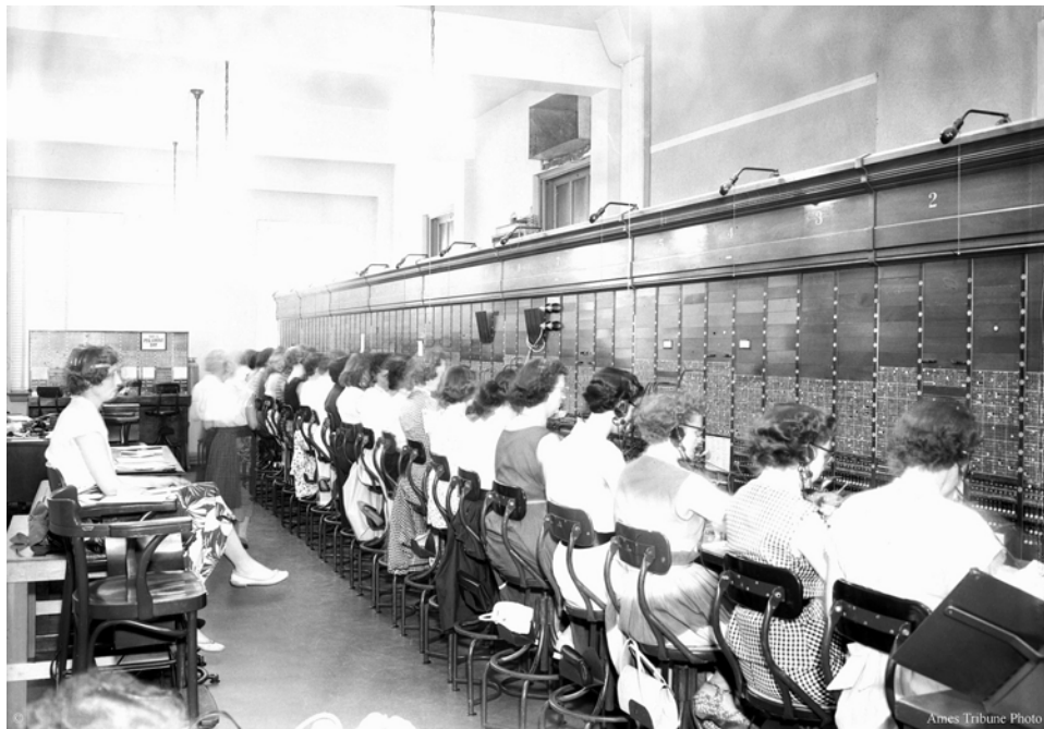
Figure 2. No. 1 common battery "A" switchboard
