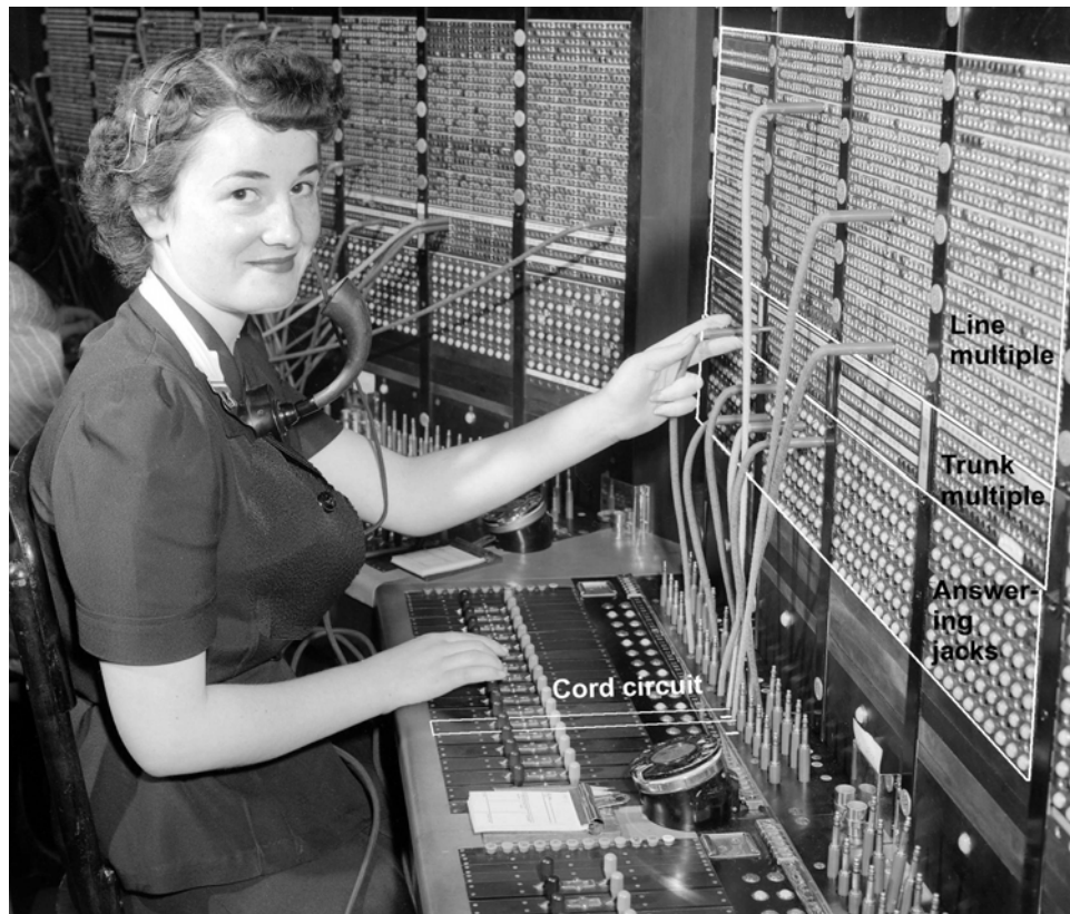
Figure 4. Automatic Electric common-battery switchboard (ca. 1947)
